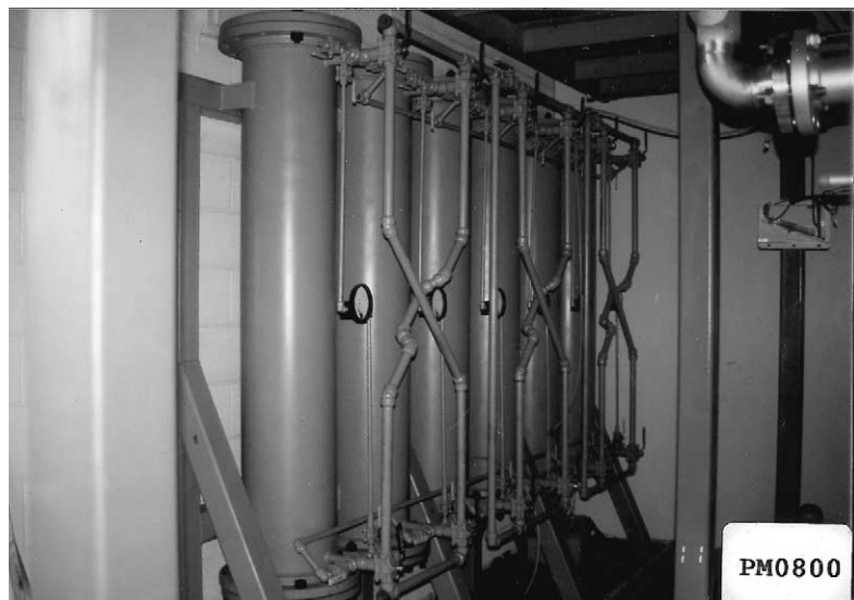
Fig. 2. FCE's desulfurization facility for 250 kW capacity natural gas clean-up.
